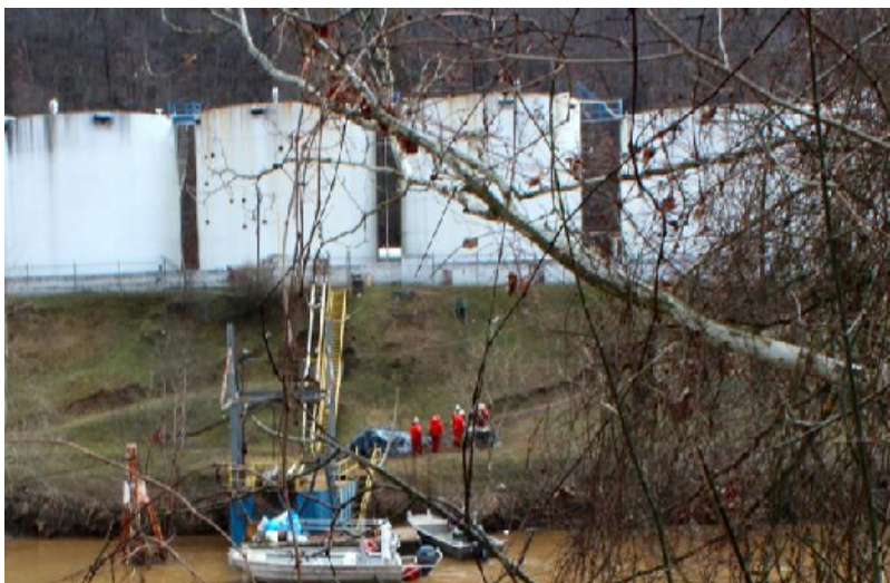
Freedom Industries tanks
