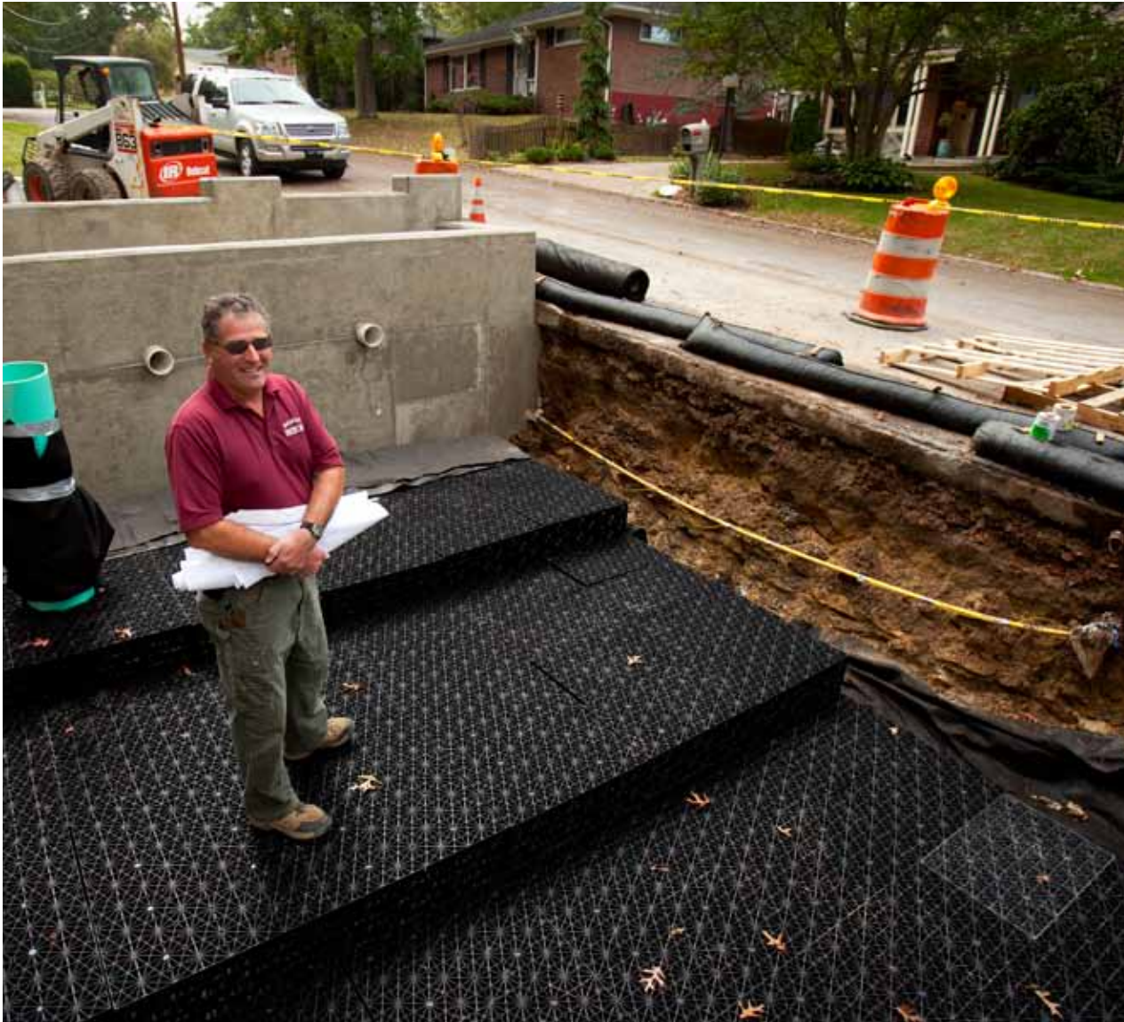
Doug King, Beckley Sanitary Board, stands on a vegetated stormwater retention system under construction in Beckley. Once complete, plants will cover the top of the facility and stormwater not taken up by the plants will filter through soil and slowly be absorbed into the ground. This system will protect houses and businesses downstream that suffer from repeated flooding.
