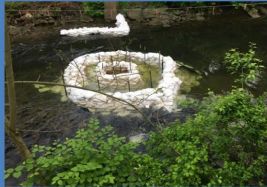
Sand bags used to contain leak of drilling fluid on Chester Creek in Brookhaven (Delaware County)
