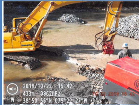
Construction continued and sediment-laden water caused violations of water quality standards in the North Fork of the South Branch of the Potomac River
