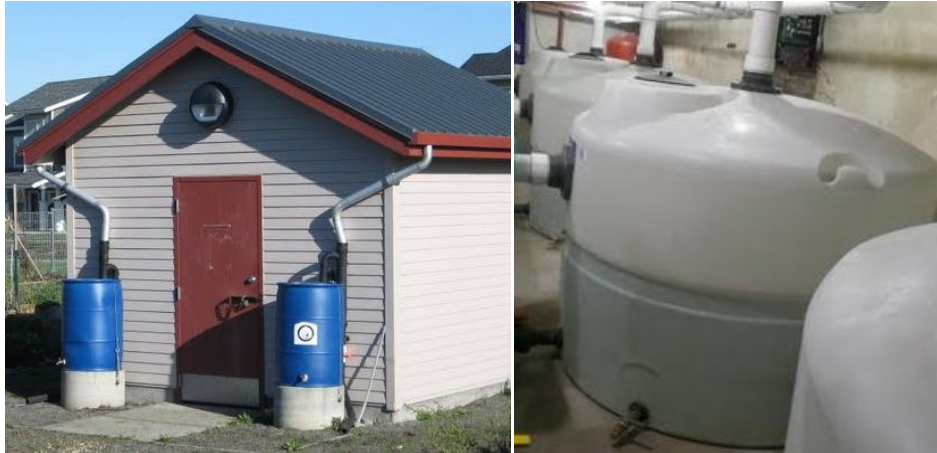
Figure 5: Rain barrels and cisterns
